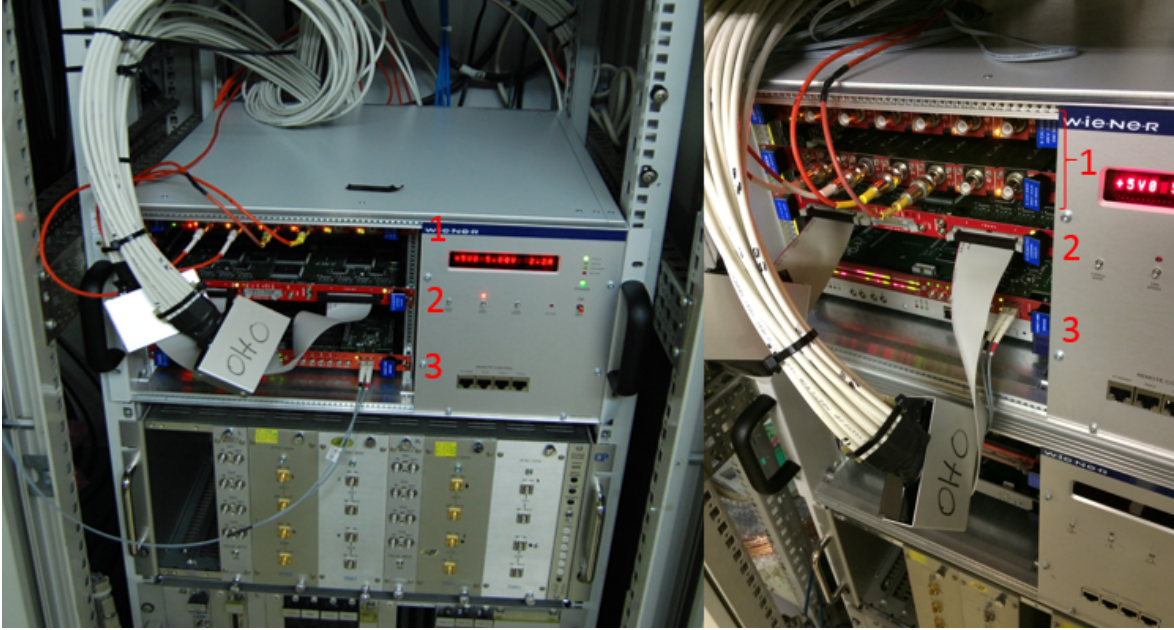
Figure 3.21: Crate for Data acquisition: 1)High Voltage (HV) CAEN V6533; 2)V830 CAEN Scaler 32 channels; 3)CAEN V2718 controller, optic fiber. A3818 pci adapter.
